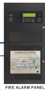
FIRE ALARM PANEL WITH SMOKE MANAGEMENT SYSTEM
